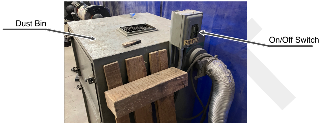
Figure 7: Front quarter view of the metal dust collection in the grinder area.
